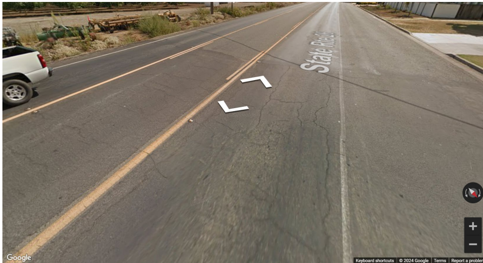
Figure 2.1: Fatigue cracking in the wheel path.
