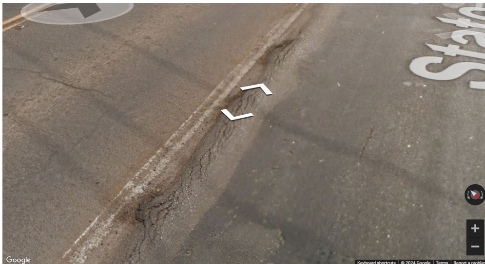
Figure 2.2: Rutting outside the wheel paths, near an intersection with farming equipment traffic.
