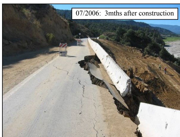
Figure 4.68: Damage associated with landslide (July 2006).
