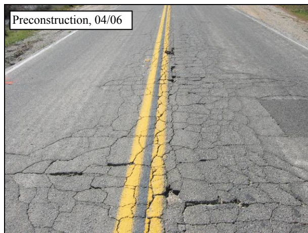
Figure 4.34: Preconstruction fatigue (alligator) cracking on 07-VEN-33.
