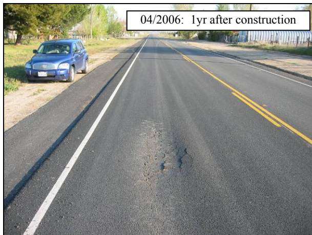
Figure 4.14: Severe distress (2) on 05-SB,SLO-33 (April 2006).
