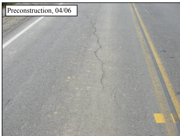
Figure 4.36: Preconstruction longitudinal cracking on 07-VEN-33.
