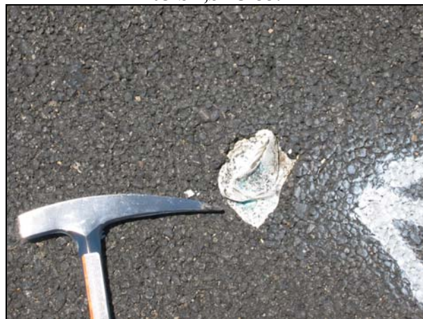
Figure 4.25: Trash compacted into asphalt concrete on 05-SB,SLO-33.
