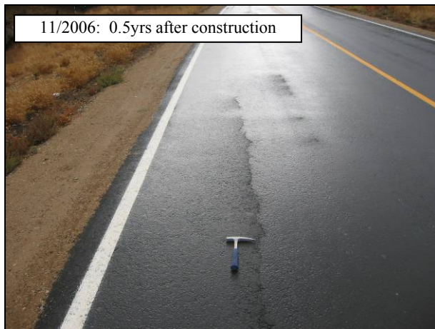
Figure 4.56: Longitudinal crack on 07-VEN-33.
