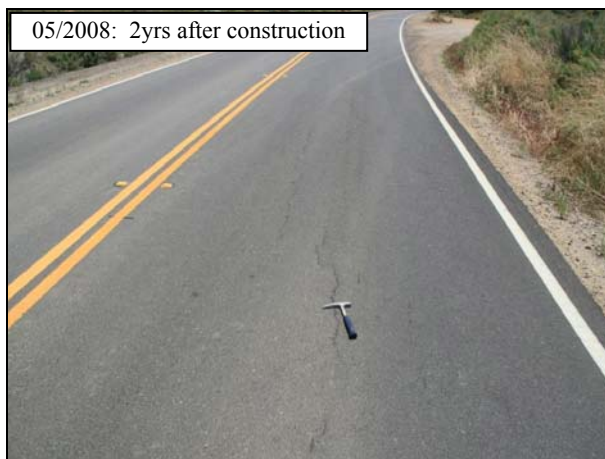
Figure 4.67: Longitudinal cracking on 07-VEN-33 (May 2008).
