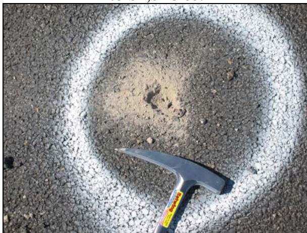
Figure 4.24: Area of thin asphalt concrete on 05-SB,SLO-33.
