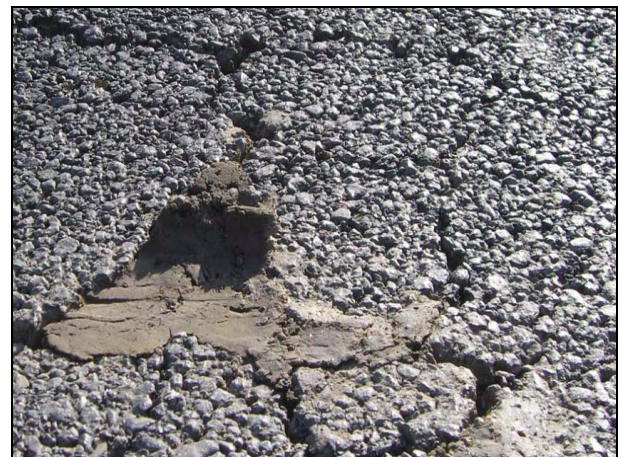
Figure 4.33: Fines pumped through base and asphalt concrete.
