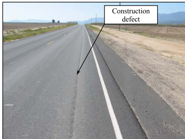
Figure 4.23: Construction defect on 05-SB,SLO-33.
