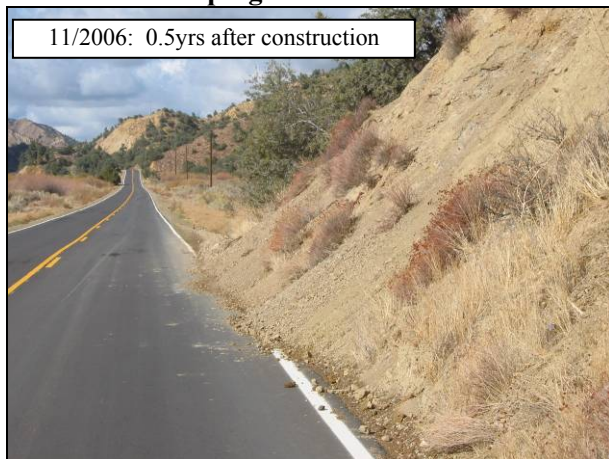
Figure 4.63: Debris from slope instability on 07-VEN-33.
