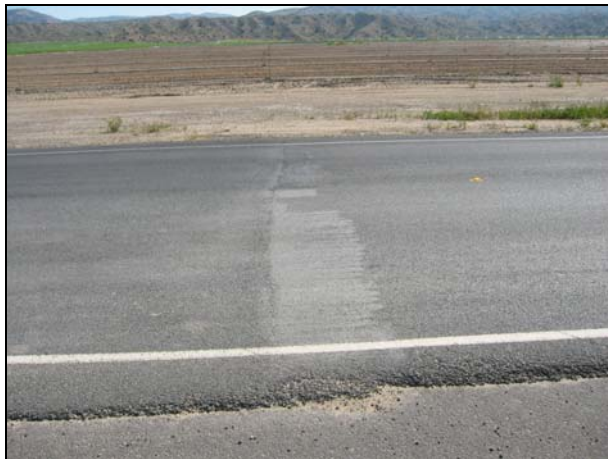
Figure 4.22: Poor construction joint on 05-SB,SLO-33.
