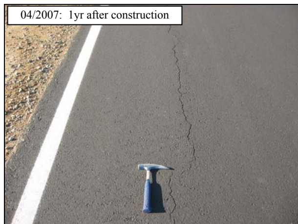
Figure 4.66: Longitudinal cracking on 07-VEN-33 (April 2007).
