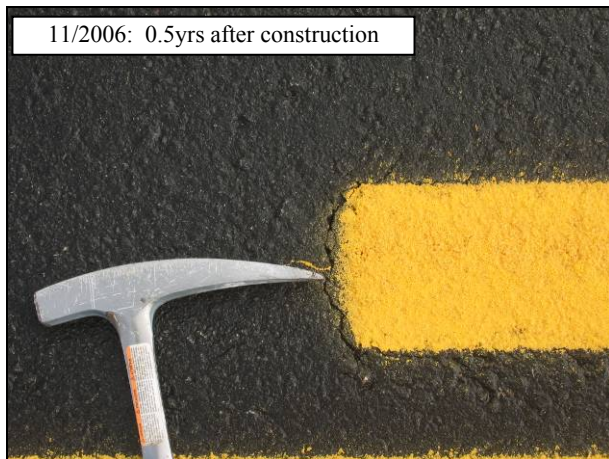
Figure 4.61: Cracking around centerline striping on 07-VEN-33.
