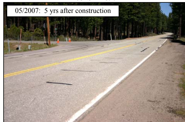
Figure 4.10: Sealed transverse cracks on 03-SIE-89.
