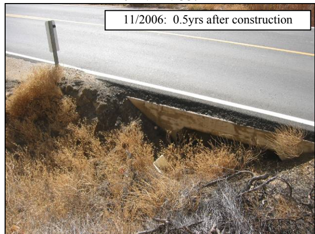
Figure 4.64: Blocked drain. (1) on 07-VEN-33.
