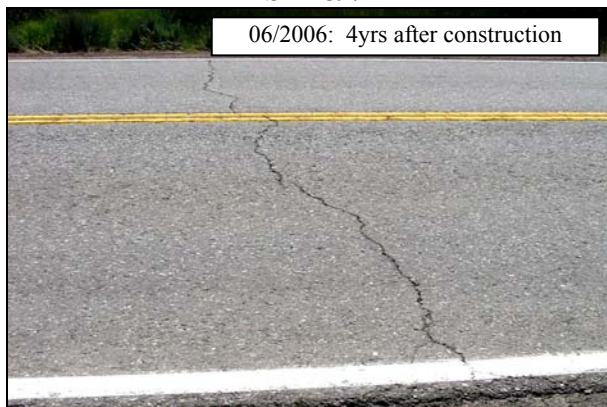
Figure 4.9: Thermal cracking on 03-SIE-89.
