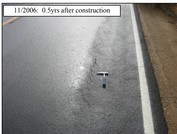
Figure 4.59: Shearing in the asphalt concrete on 07-VEN-33.
