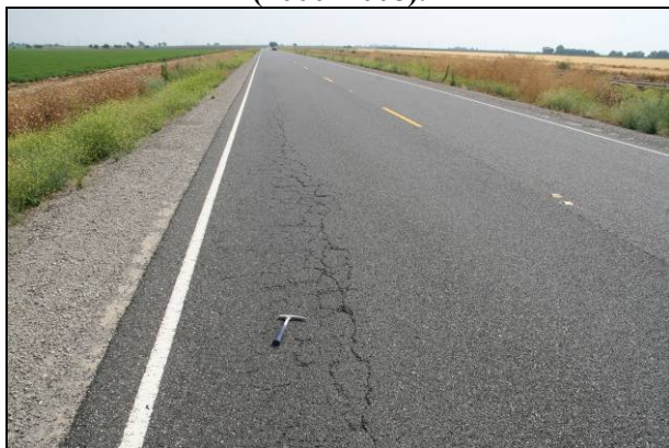
Figure 4.4: Fatigue cracking in outer wheelpath on 03-COL-20 (2008).
