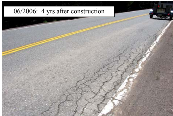
Figure 4.7: Outer wheelpath cracking on 03-SIE-89.
