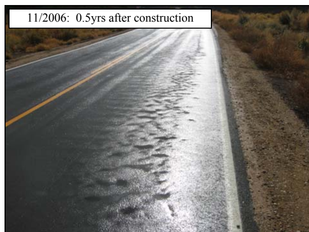
Figure 4.60: Roughness in asphalt concrete on 07-VEN-33.
