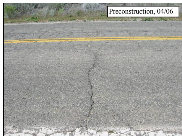
Figure 4.35: Preconstruction transverse cracking on 07-VEN-33.
