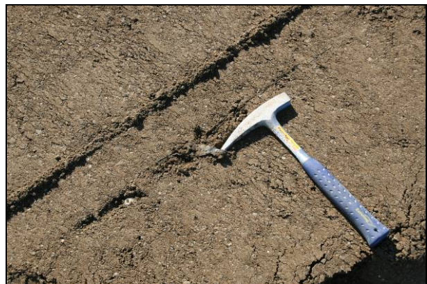
Figure 7.31: Asphalt strings in recycled material.
