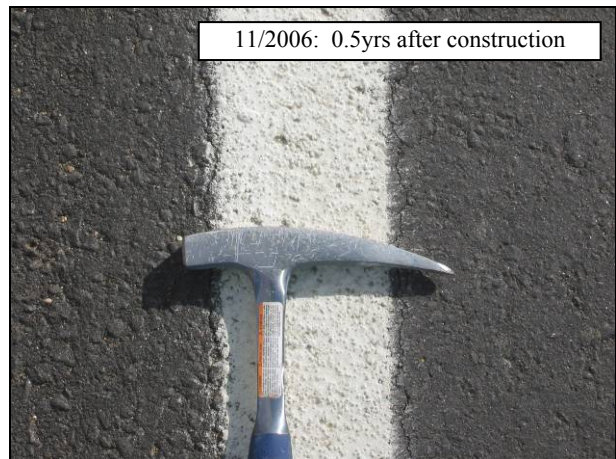
Figure 4.62: Cracking around edge striping on 07-VEN-33.
