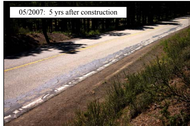
Figure 4.8: Sealed outer wheelpath cracks on 03-SIE-89.
