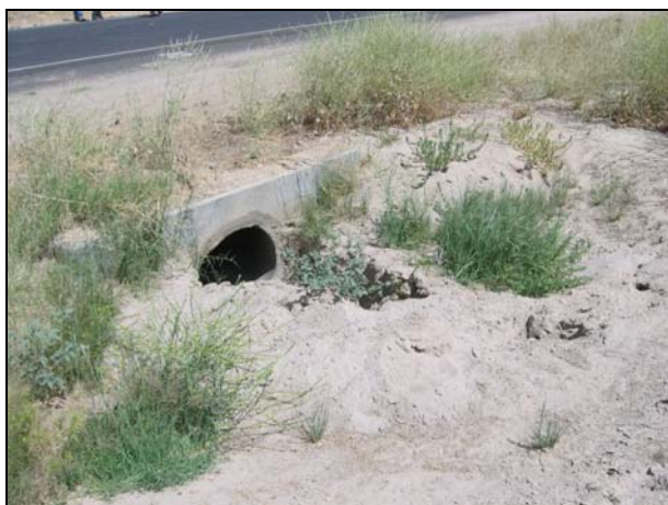
Figure 4.19: Blocked culvert on 05-SB,SLO-33.
