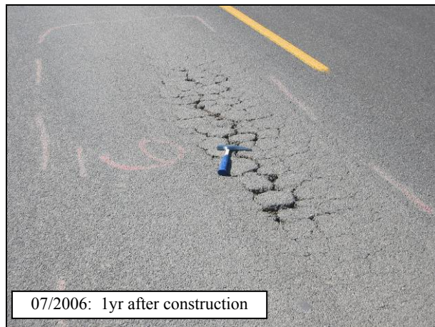
Figure 4.15: Severe distress (3) on 05-SB,SLO-33 (July 2006).
