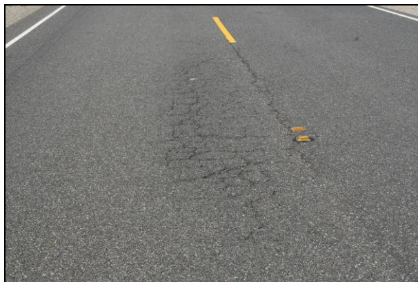
Figure 4.3: Fatigue Cracking in inner wheelpath on 03-COL-20 (2007).
