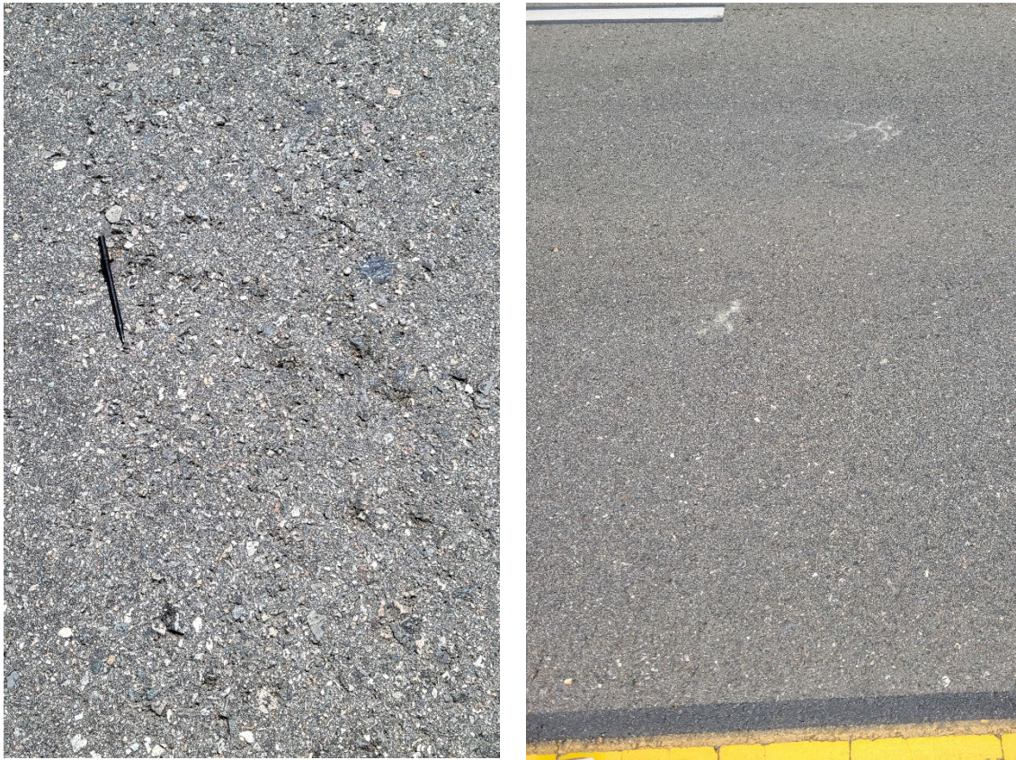
Figure 3.8. Slight aggregate loss at PM 14.21 and pumping at PM 14.40 in the 35% RAP mix southbound.
