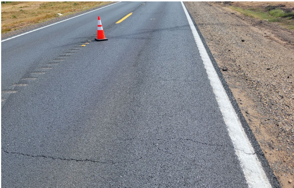
Figure 3.14. Example of transverse cracking in the 40% RAP mix at PM 8.78.
