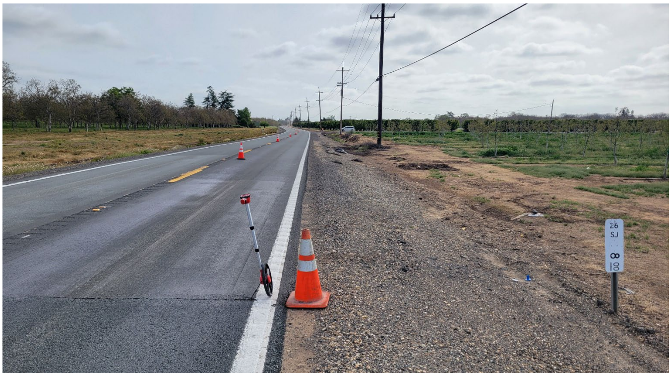
Figure 3.12. Transverse cold joint at beginning of SJ 26 test sections eastbound at PM 8.0.
