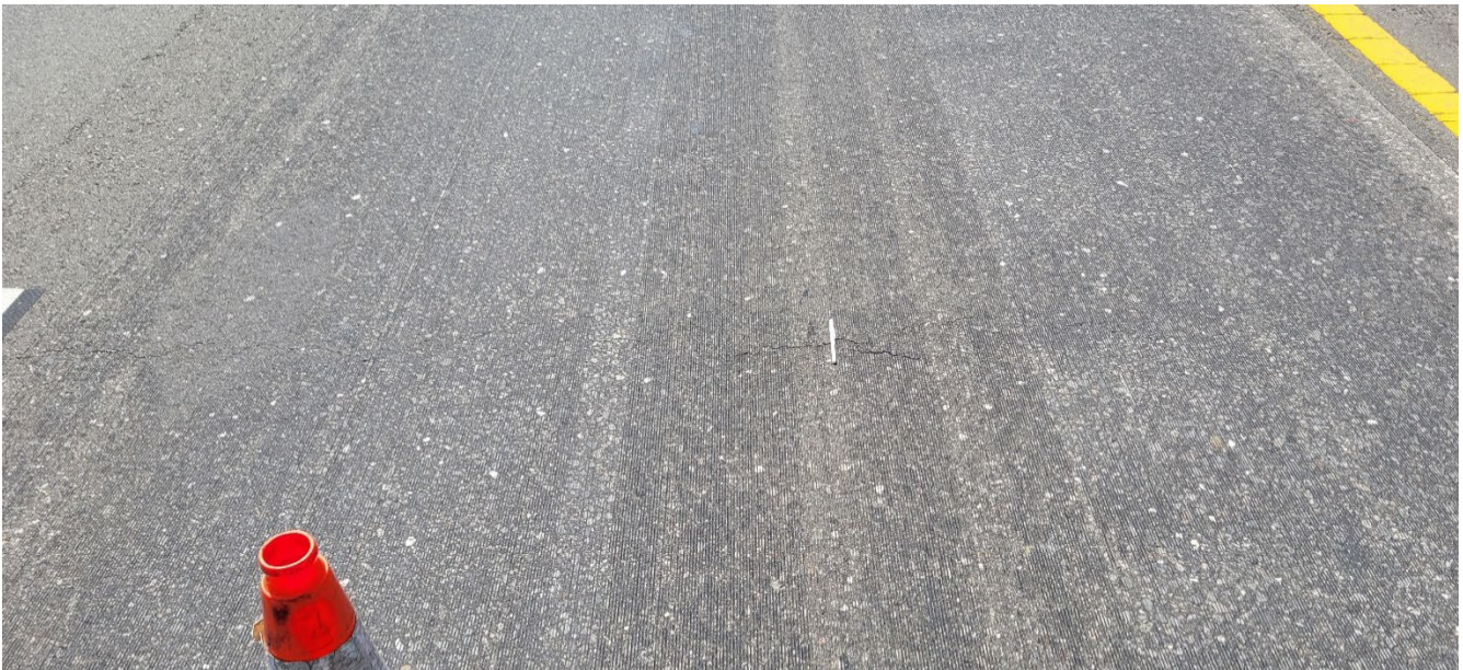
Figure 3.6. Transverse crack near SBD 215 northbound at PM 15.00.
