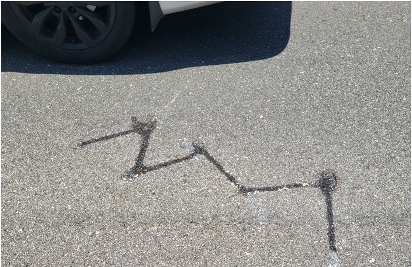
Figure 3.10. Burn marks on surface in southbound direction between PM 14.0 and PM 15.0.
