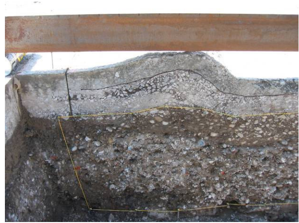
Figure 3.53: 589RF#12 severe displacement on edge of rut.
