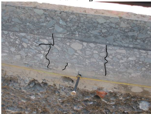
Figure 3.66: 591RF cracks in underlying DGAC.
