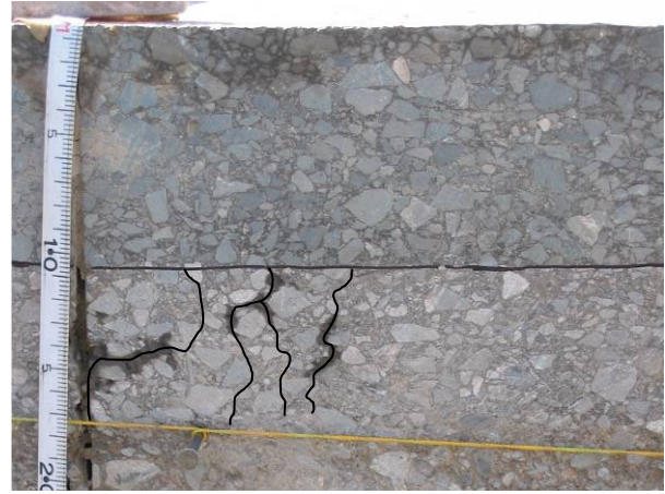
Figure 3.59: 590RF cracks in DGAC layer.
