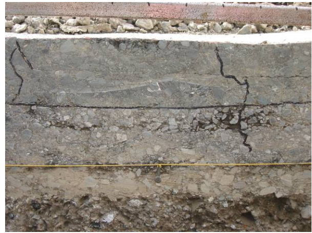
Figure 3.47: 588RF cracks in overlay and underlying DGAC.
