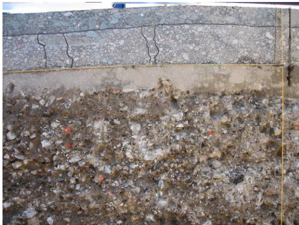
Figure 3.38: 587RF#4 cracks in underlying DGAC.
