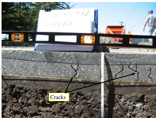
Figure 3.32: 586RF cracks in underlying DGAC.
