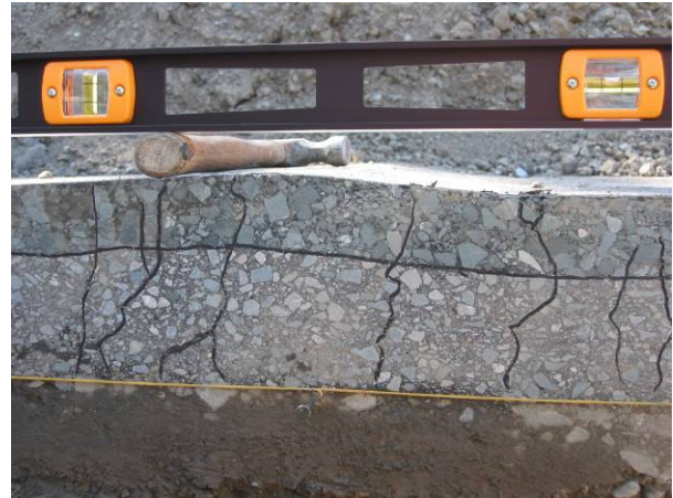
Figure 3.37: 587RF#4 cracks in overlay and underlying DGAC.
