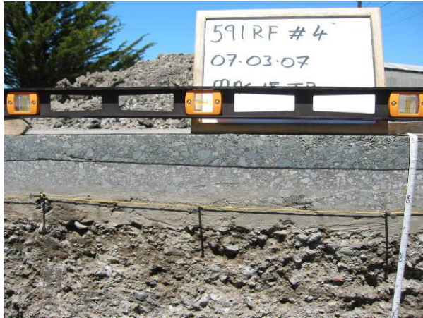
Figure 3.64: 591RF#4 rutting from Phase 1 trafficking.
