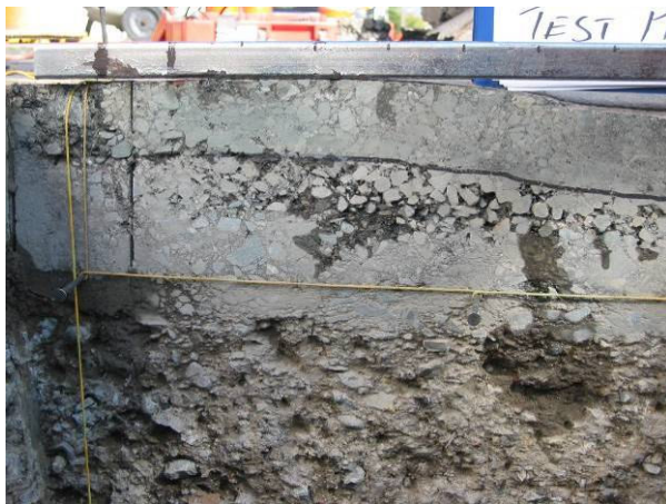
Figure 3.10: 581RF segregation in DGAC layer.
