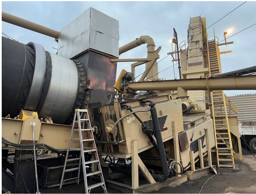
Figure 2.3: Pug mill for mixing RAP and recycling agent.
