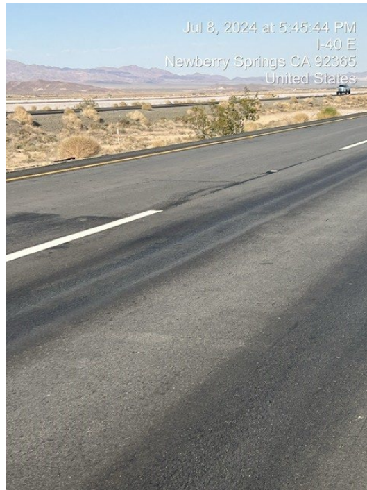
Figure 6.1: Rutting in July 2024 in Lane 2 of HyRAP test section.
