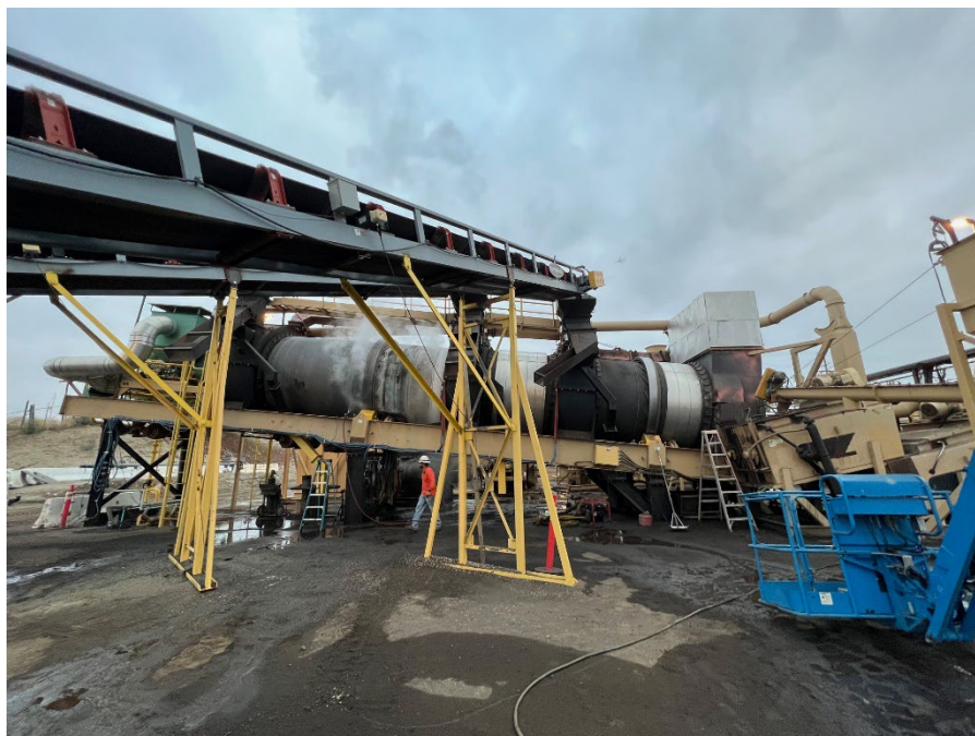
Figure 2.2: Dryer drum for drying and heating RAP.
