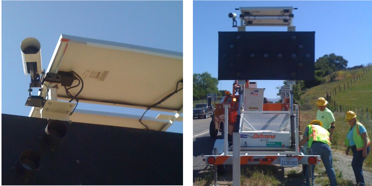
Figure 4: Camera and Solar Panel
