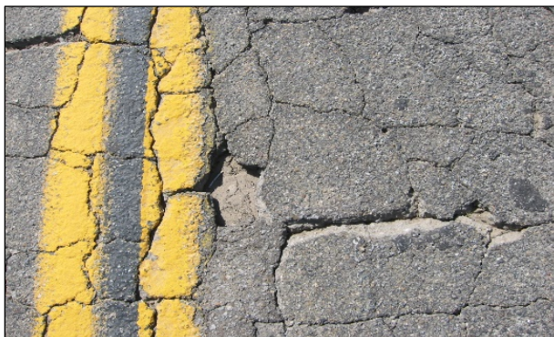
Figure 2.23: Example bottom-up distresses: Unsealed reflective cracks.
