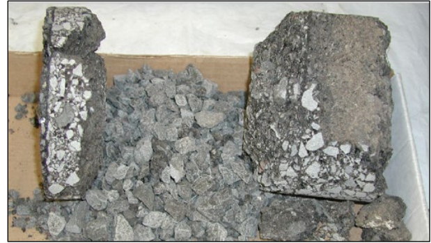
Figure 2.48: Stripped asphalt concrete layer.
