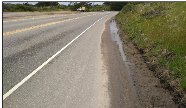
Figure 2.7: Example drainage problem in cut.
