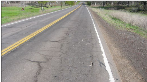
Figure 2.19: Example bottom-up distresses: Fatigue (alligator-B) cracks.
