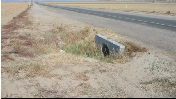
Figure 2.33: Blocked side drain and culvert.
