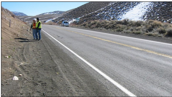
Figure 2.37: Absence of drains below cut slopes.
