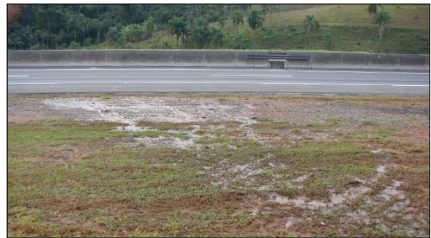
Figure 2.38: Water flowing downslope into the road.
