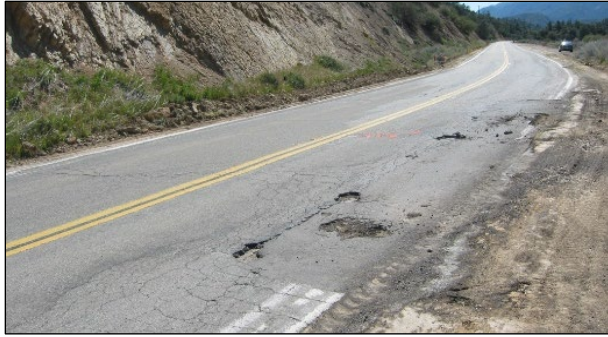
Figure 2.17: Example top-down distresses: Potholes.
