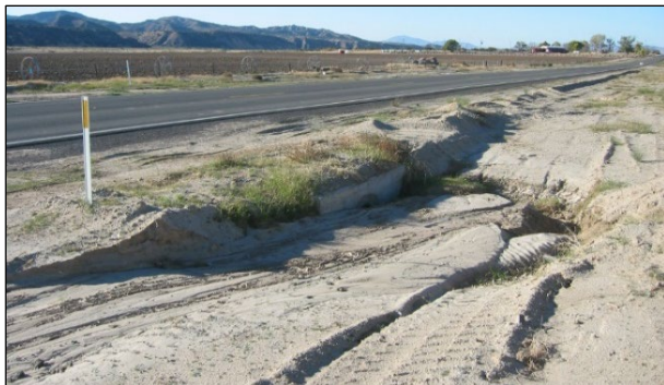
Figure 2.6: Example blocked side drains and culvert.
