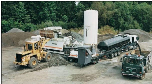
Figure 6.10: Cold central plant.
