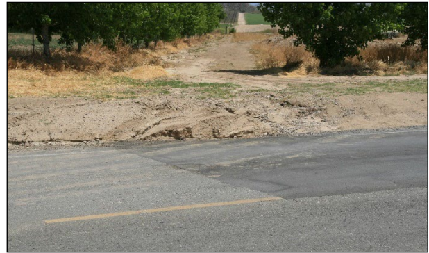
Figure 2.36: Access road drainage problems (note patch).
