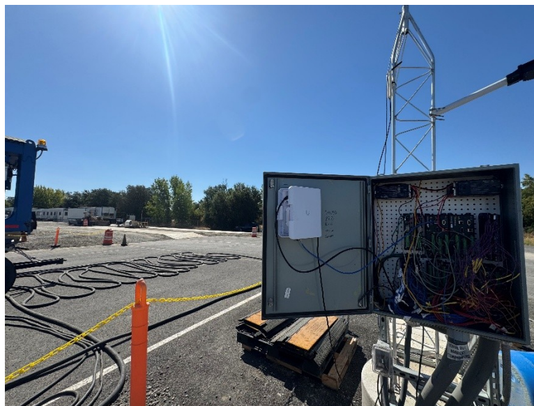
Figure 3.26: Data acquisition system (DAS) box by the slabs.
