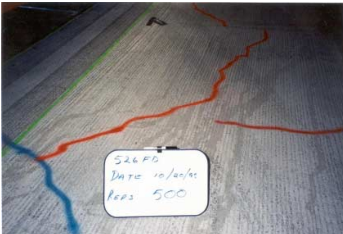
Photograph 4.29. Crack pattern after 500 repetitions, Test Section 526FD.
