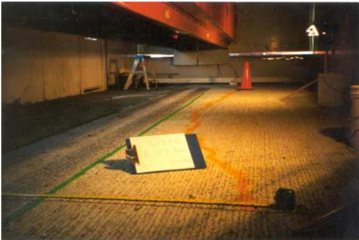
Photograph 4.2. Longitudinal crack after 2,105 repetitions, Test Section 519FD.
