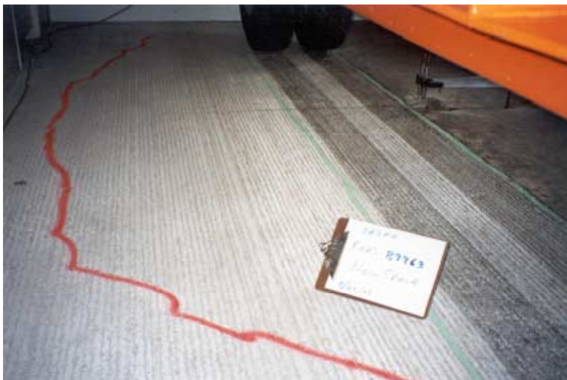
Photograph 4.23. Crack pattern after 90,000 repetitions, Test Section 523FD.
