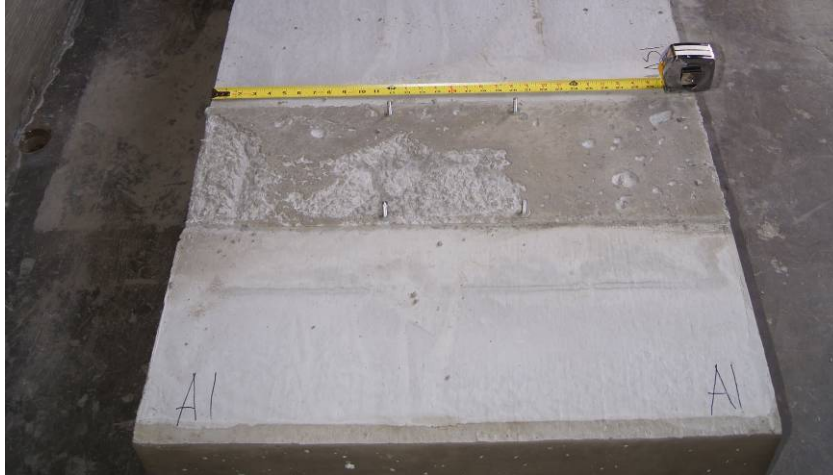
Figure 5-14: Uneven raised surface at cast-in anchor locations
