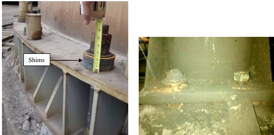
(a) Chimney base connection with ~2 in. of anchor stretch (shims placed after event)
