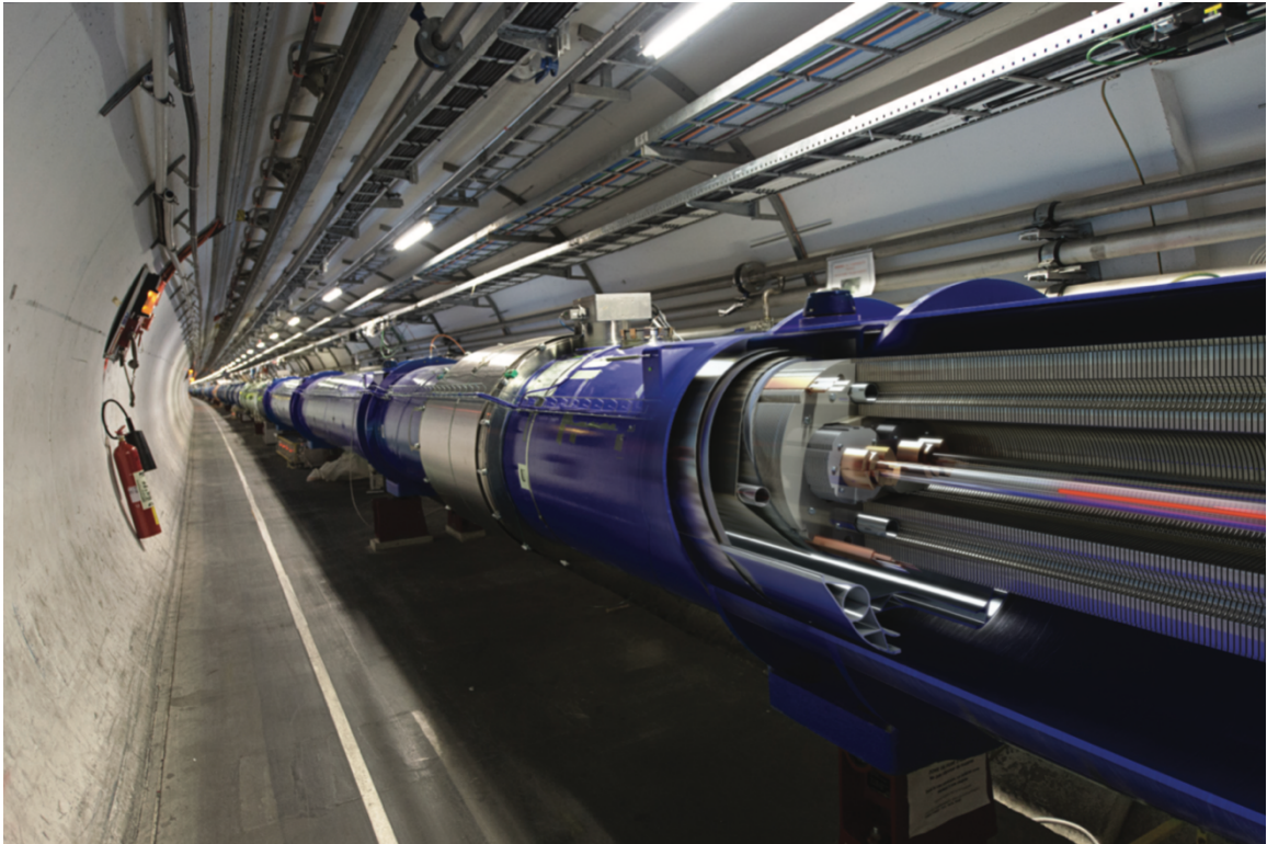
Figure 2-3: The LHC tunnel, with cutaway view of the dipole magnet. This image is taken from [65]
