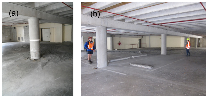
Figure 4.8.5. Photos of the ground floor level of the SCH building. While significant sediment ejecta was observed, there was little differential settlement.
