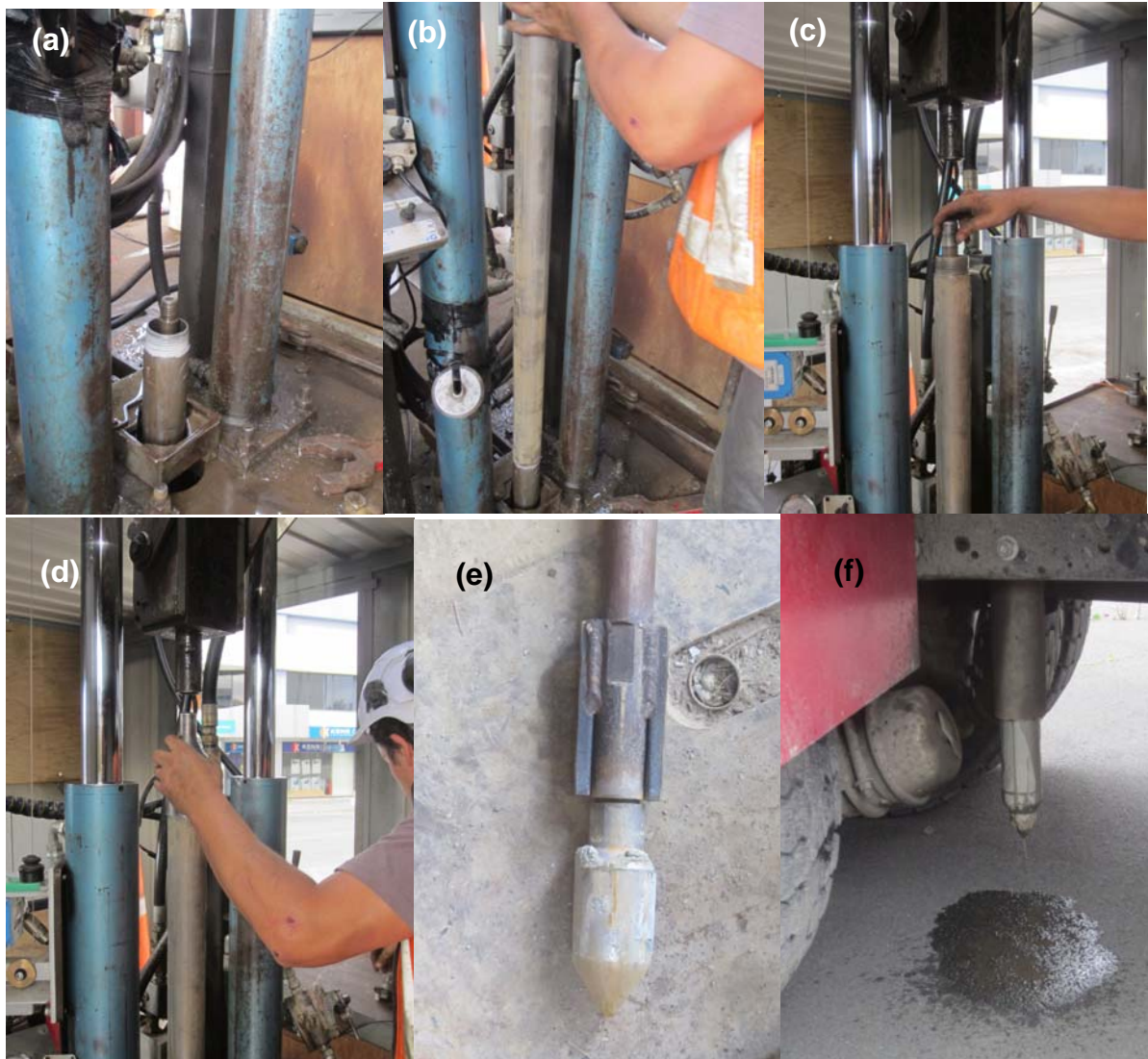
Figure 4.1.20. (a) View of dual tube casing system. (b) Connecting additional casing rods. (c) View of casing rods prior to driving cap placement. (d) View of casing rods following driving cap placement. (e) View of inner rod tip. (f) View of tip of casing assembly through the CPT truck sleeve prior to shallow driving.
