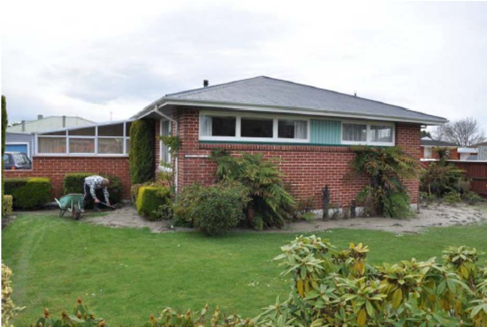
Figure 2.2.6. Example of residence in Kaiapoi subjected to liquefaction-induced ground movement during the September 4, 2010 M_w 7.1 Darfield earthquake. Note the liquefaction-induced sediment ejecta around the perimeter of the foundation. This house experienced approximately 40 cm of settlement along the north side (from Green et al., 2010).
