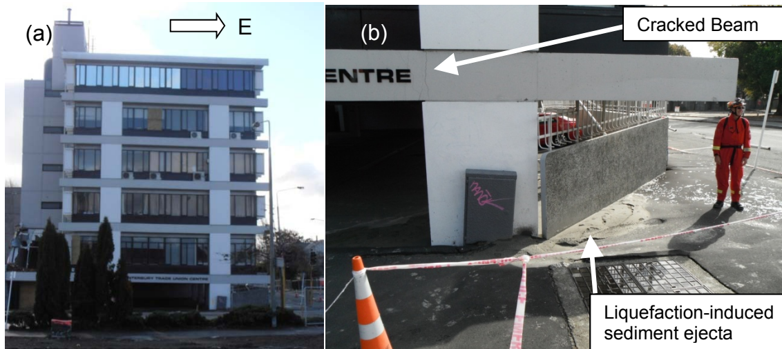
Figure 4.3.5. (a) South end of CTUC Building showing tilt to the east (taken July 2011) and (b) Close-up photograph of the SE corner of the building (taken March 2011).
