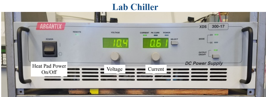
Figure 7.4: The front panel of the Argantix heat pad power supply. The on/off switch is the most commonly used and the displays for the voltage and current are checked constantly but not controlled by the knobs on the front panel
