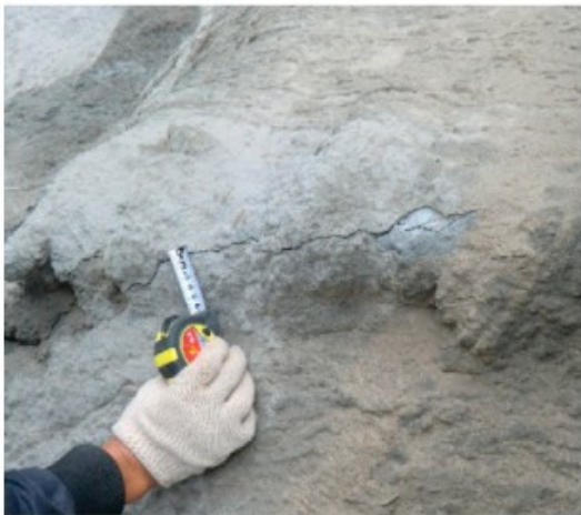
(c) Crack C on the cut slope.
