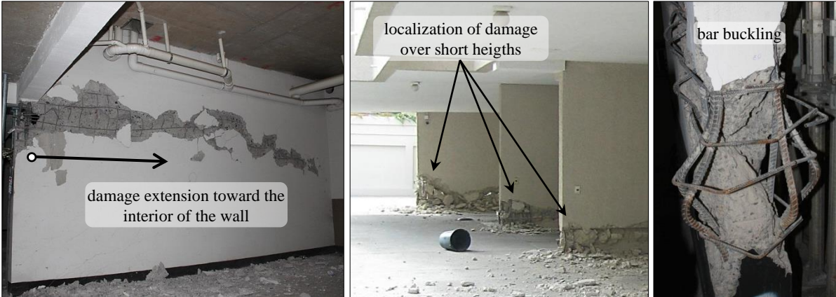
Figure 1.1 - Observed damage in multistory reinforced concrete shear wall buildings during the 2010 Maule Earthquake in Chile [center: 10-story building in Viña del Mar (photo by Patricio Bonelli); right: 19-story building in Santiago (left and right photos by Jack Moehle)]
