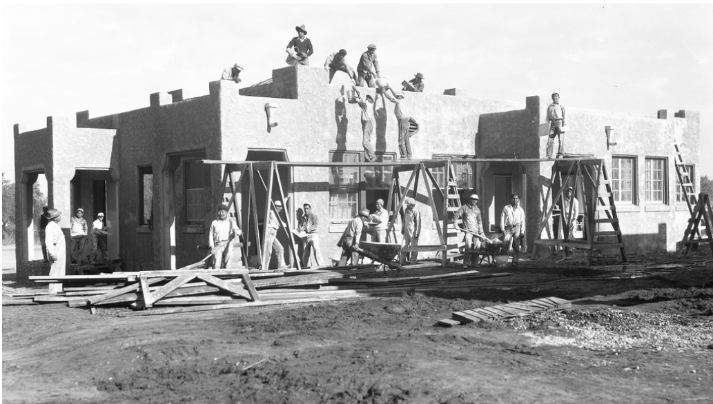
Figure 17: Construction photos, before and after the plaster façade is applied to the new shop building by students at the Sherman Institute, ca. 1930-40, Box 150&154, SIM
