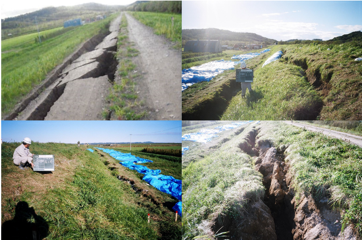
Figure 4.26 Damage at Section 12, cracks on the roadway on the levee crest (top left). Slip and displacement of the land-side slope towards the levee toe (top right, bottom).
