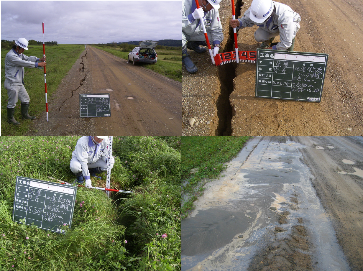
Figure 4.16 Cracking on the crest (top) and land-side slope (bottom left) at Section 8. Sand boils on crest access road downstream (bottom right).
