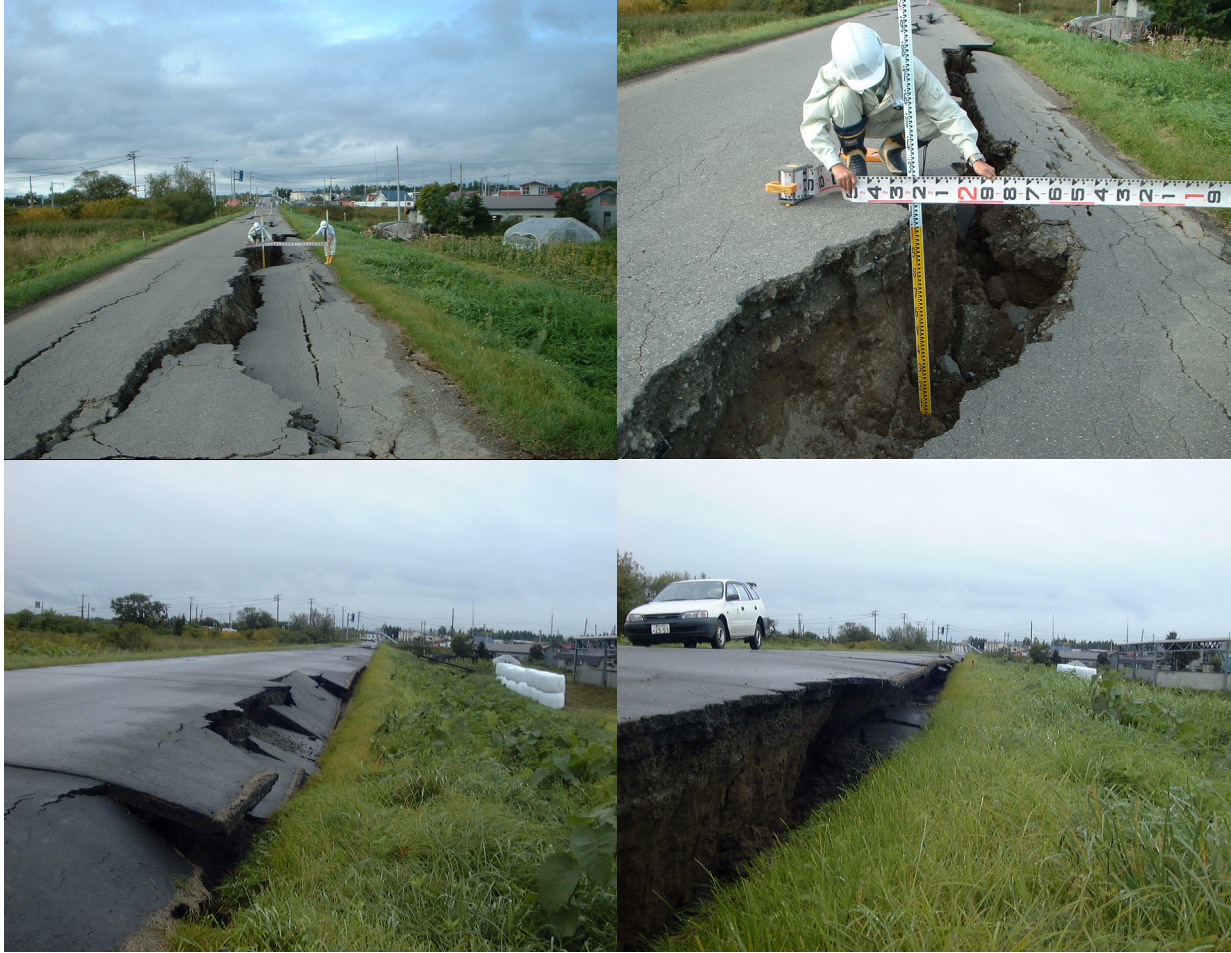
Figure 4.31 Cracks on the roadway on the levee crest at Section 14 from slip on land-side slope.
