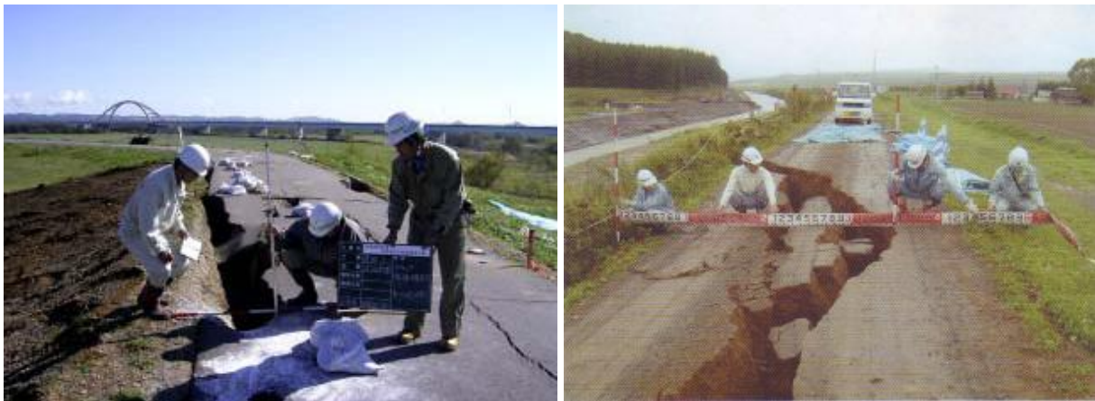
Figure 4.21 Cracking of the roadway on the levee crest accompanied by slip on the slope at Section 10.
