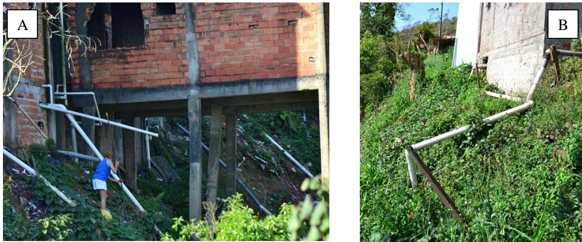
Figure 3.7. 7A and 3.7B. Fig. 3.7A. Precarious wastewater pipes and pipes to conduct water. Fig. 3.7B. Self built pipelines. Note black tape to help keep pipes connected.
