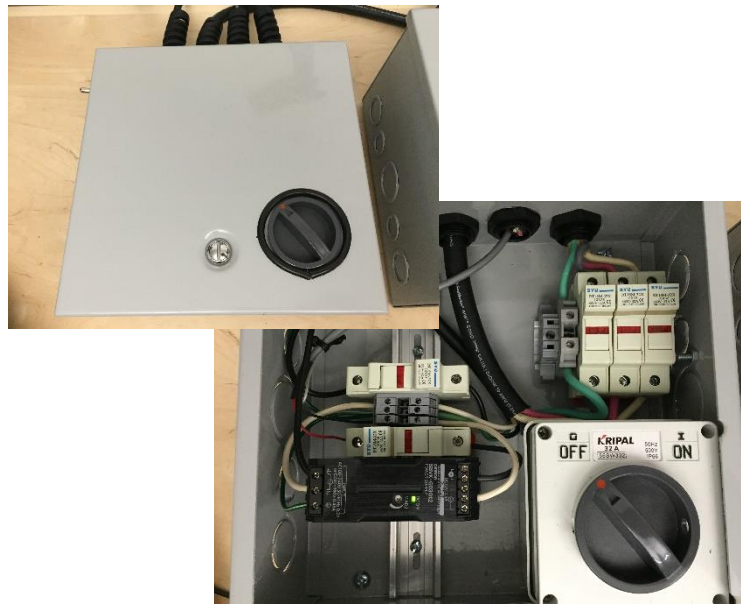
Figure 2-23: All fuse blocks, power switches, and the DC power supply are housed in a junction box.
