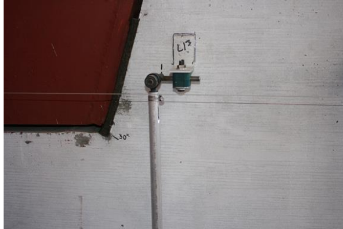
Figure 6.57 First crack on the east face of shear key 9A
