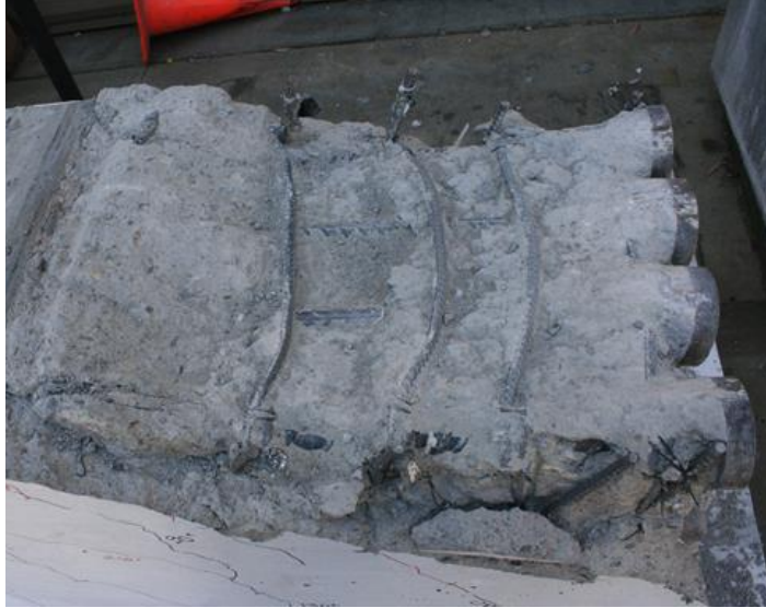
Figure 6.77 Sliding plane surface after shear key 9B was removed
