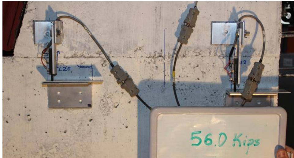
Figure 5.36 Construction joint condition at 56 kips for shear key 7B
