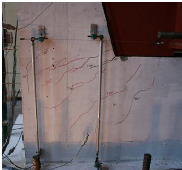
Figure 6.88 Crack behind the horizontal shear reinforcement of the stem wall on the west face of shear key 10A
