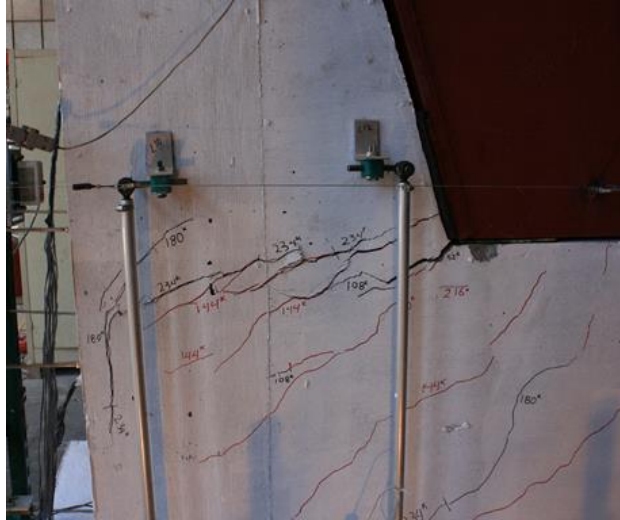
Figure 6.89 Diagonal cracks join to form a sliding plane on the west face of shear key 10A
