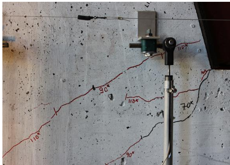
Figure 6.31 Change in the direction of crack propagation on the west face of shear key 8A
