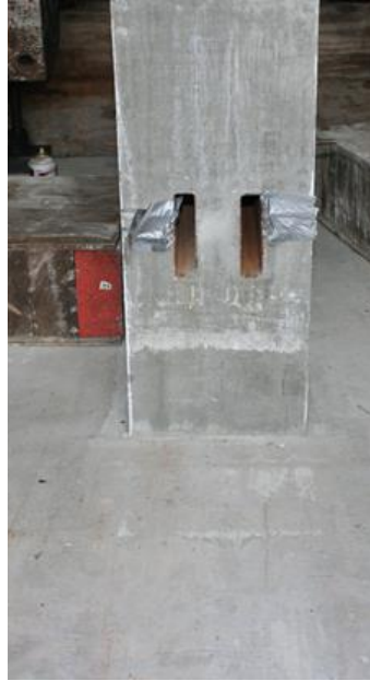
Figure 7.38 Stem wall and footing after shear key block was removed in Test 5
