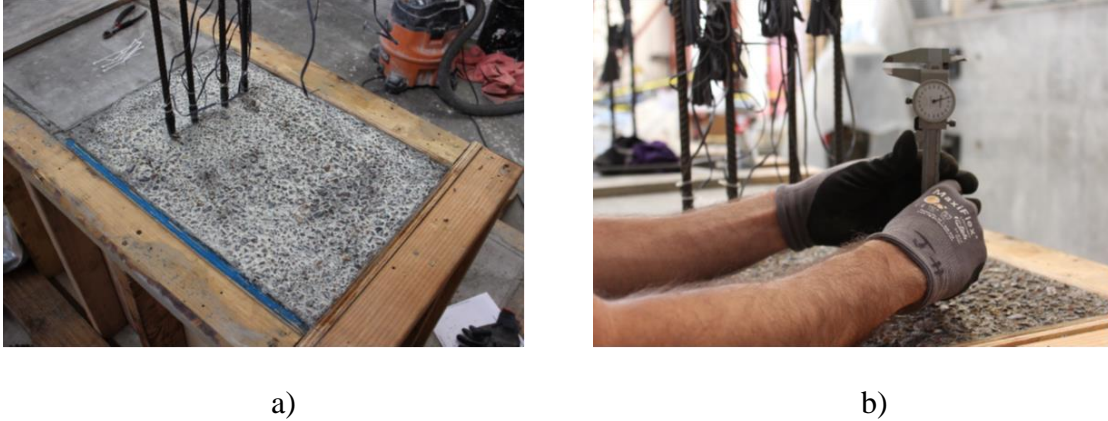
Figure 5.6 Construction joint of shear key 7B: a) roughened surface; b) roughness measurement
