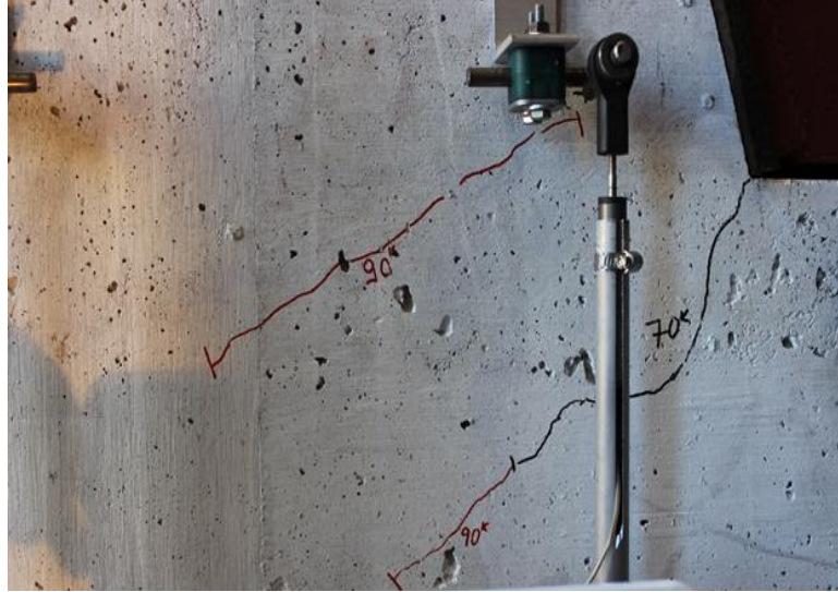
Figure 6.30 Propagation of diagonal crack and formation of additional diagonal crack on the west face of shear key 8A
