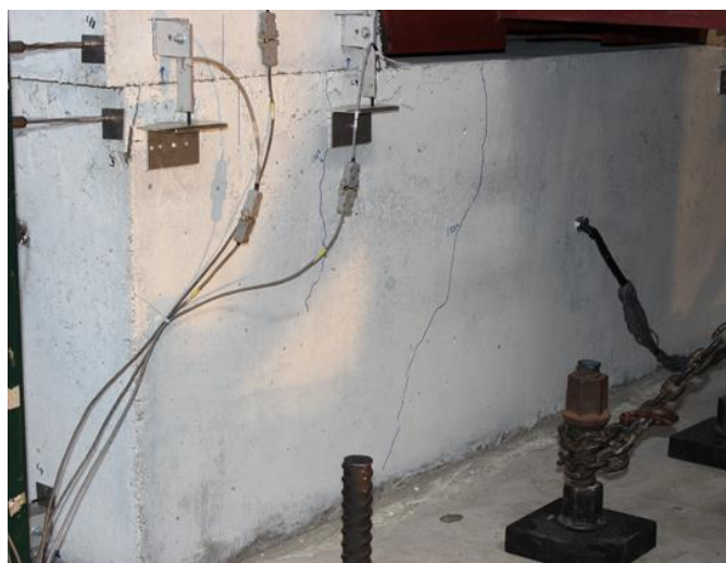
Figure 5.24 First two cracks observed on the east face of shear key 7A
