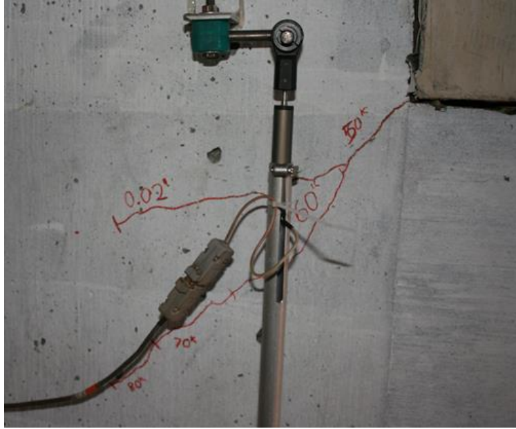
Figure 6.46 First horizontal crack on the east face of shear key 8B
