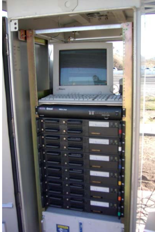
Figure 1.2 V2DVS Data Acquisition Computers in Type 334 Cabinet, Testbed Site at Sand Canyon Overcrossing.
