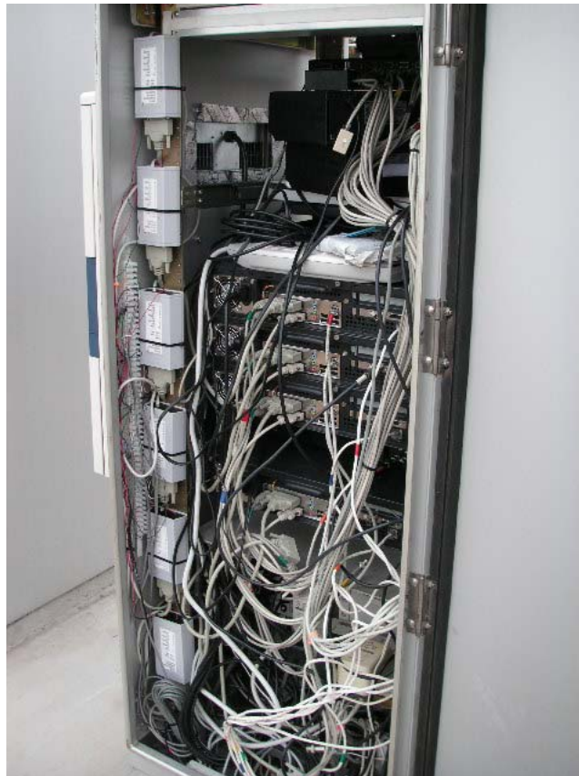
Figure 12.1. Contact-closure interface boxes for each lane, mounted on back left rail of 334 cabinet.
