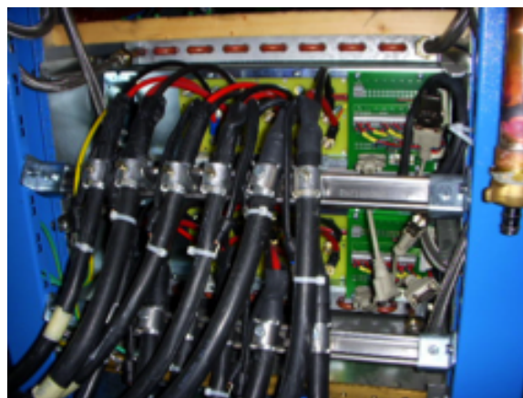
Figure A.3: The back of a maratón with 4.5 V and 6.5 V cables connected is shown. Metal rails attached to the electronics rack (blue) can be seen along with metal brackets that securely hold the black cables in place.
