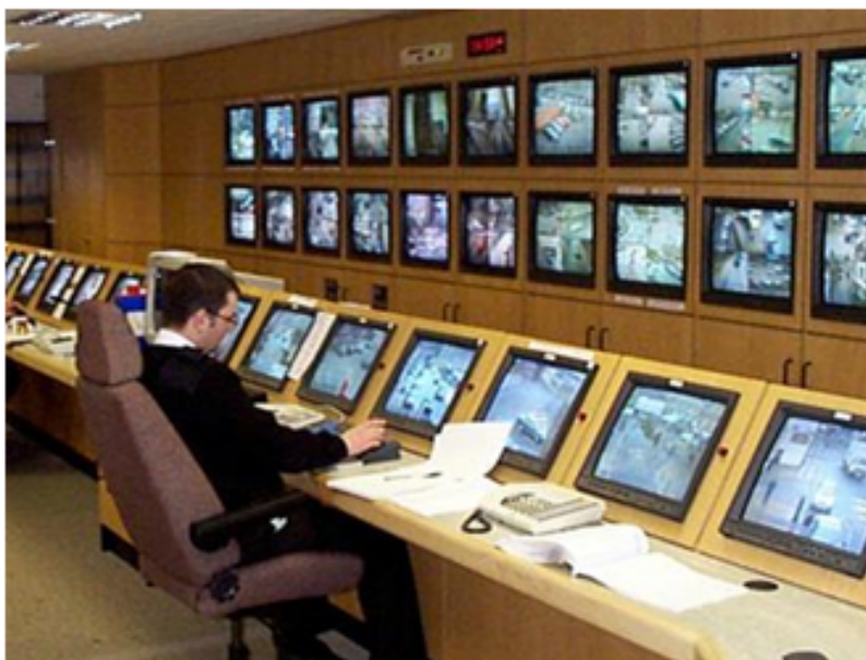
Figure 4.1: Typical CCTV control room with video feeds from several cameras
