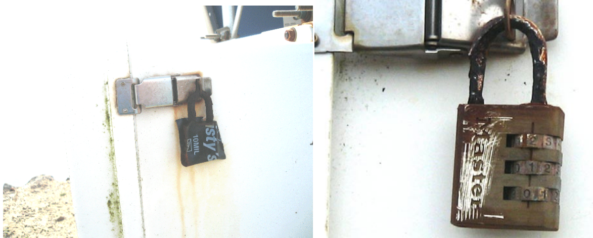
Figure 36. Padlocks on enclosure boxes showing level of rust and corrosion after 18 months exposure to salt environment. Left is at Point Reyes Lighthouse Rock, right is Point Reyes RCA Building. Locks had to be forcibly removed with saw.
