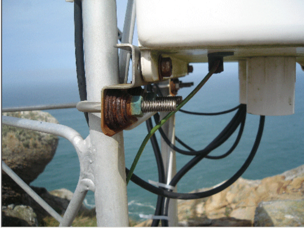
Figure 35. Point Reyes Lighthouse Rock station, showing corrosion of steel bolt after 18 months of exposure to salt. Site is 526 feet directly above the Pacific Ocean.
