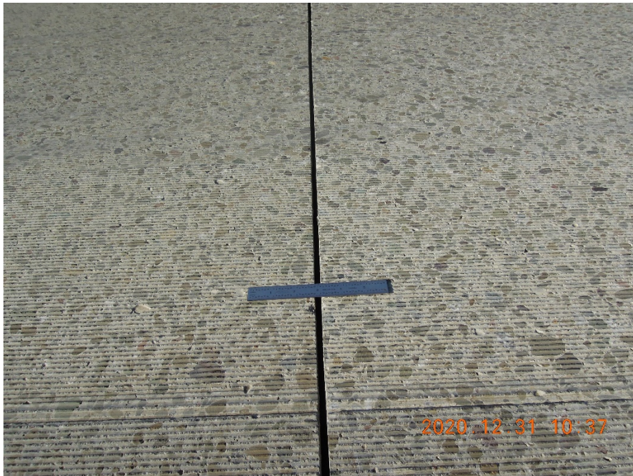
Figure 4.2: No faulting at transverse joint.
