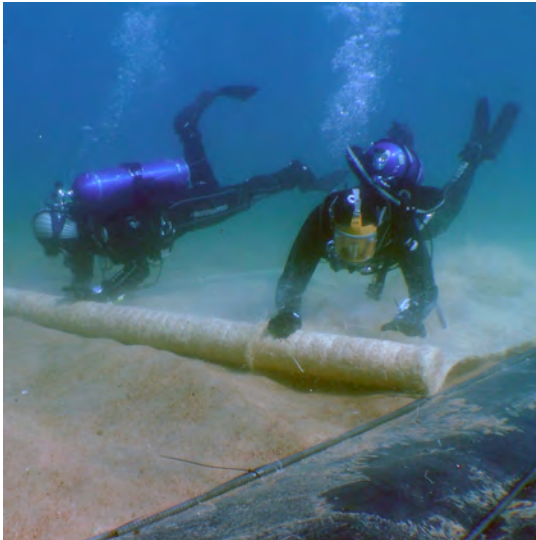
Figure 3-2. Divers rolling out mats made from aspen shavings (see “Success Story”). Photo Credit: Jim Brockett, Tahoe Resource Conservation District
