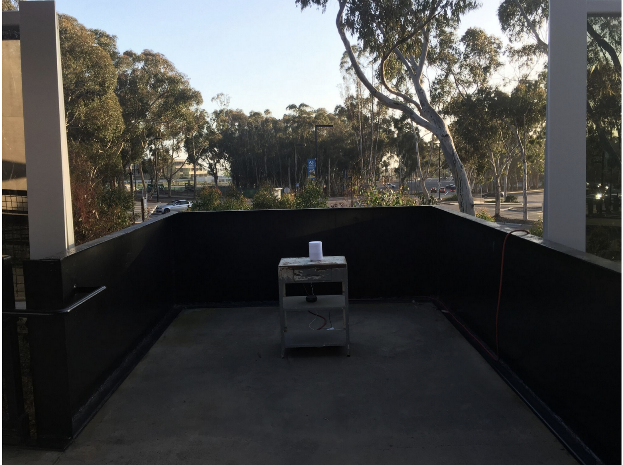
Fig. 3.5: Far view of the balcony protrusion. Note the glass wall on the peripheries.
