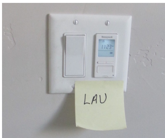
Figure 16: Programmable Controller Used to Control Exhaust Ventilation in Laundry Room
