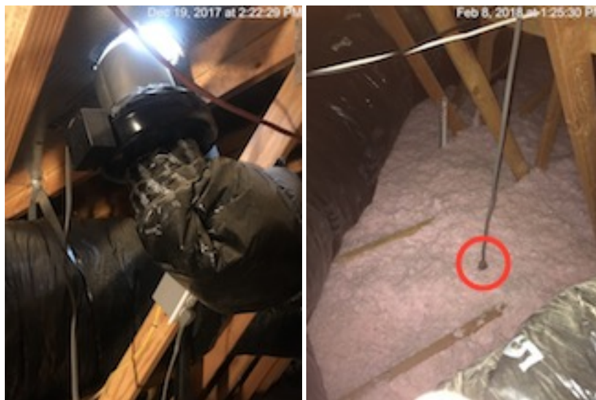
Observed installation problem: (left) exhaust fan detached from roof, (right) exhaust fan not plugged in.
