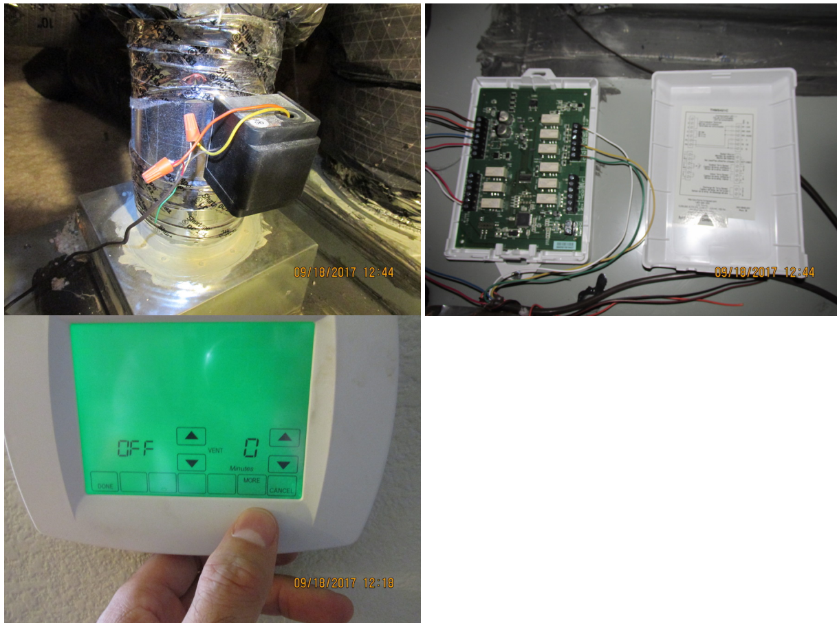
(top left) CFIS motorized damper and (top right) control module. (bottom) Thermostat showing ventilation control option was turned off.
