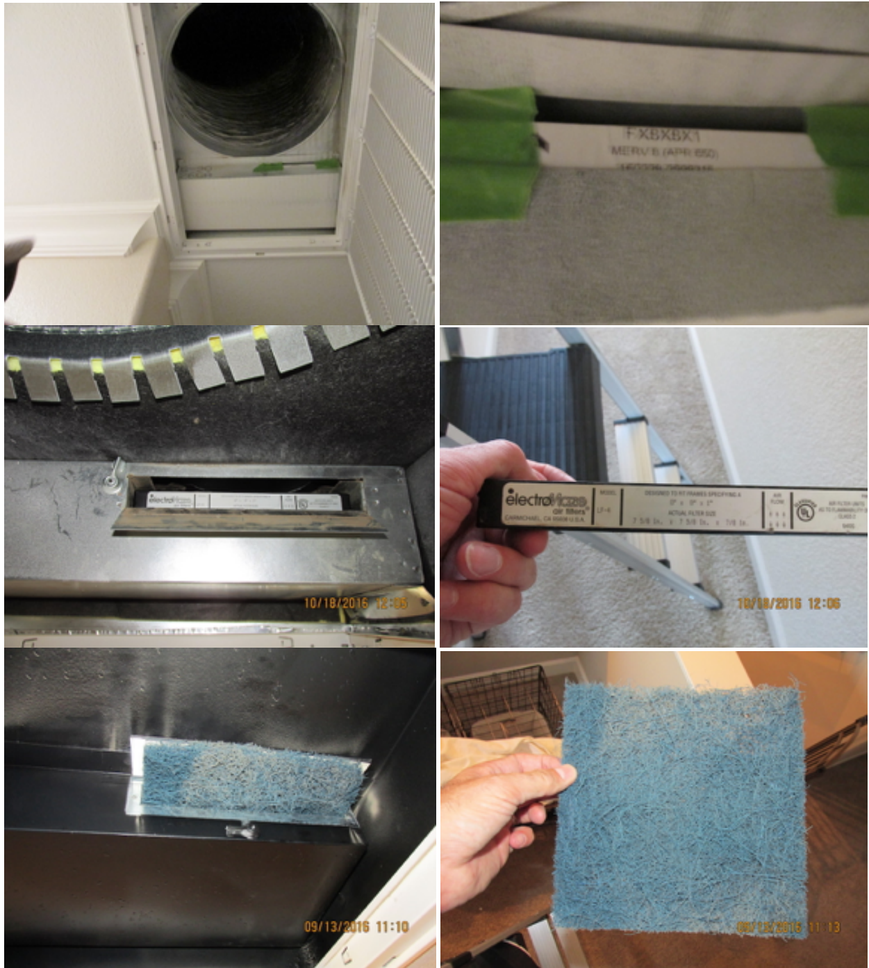
Photos of the supply air filter used in three homes.
