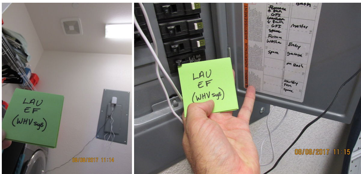
Figure 10: Continuous Exhaust Ventilation Controlled at Breaker Panel in One Home
