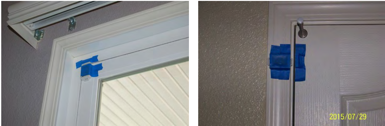
Figure 6 State logger used to monitor opening and closing of windows and doors.
