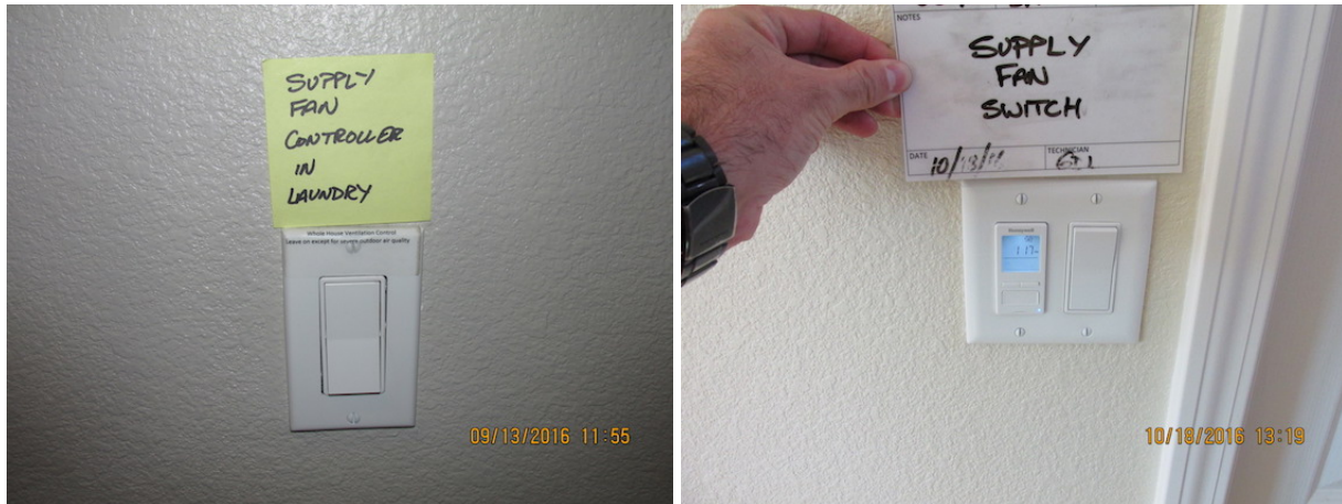
(left) Label reads: “Whole House Ventilation Control. Leave on except for severe outdoor air quality”. (right) Programmable controller used to control inline fan for supply ventilation.
