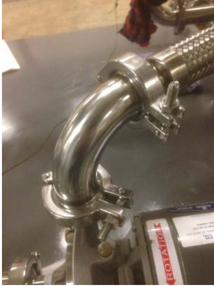
Figure 3-13: Tri-clamp fittings from the pump discharge to the flexible stainless steel tubing going to the heater
