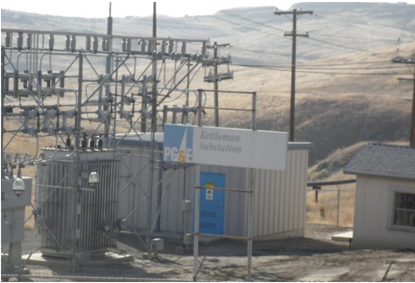
PG&E Kettleman Substation located near Avenal. Photograph by Daisy Lopez
