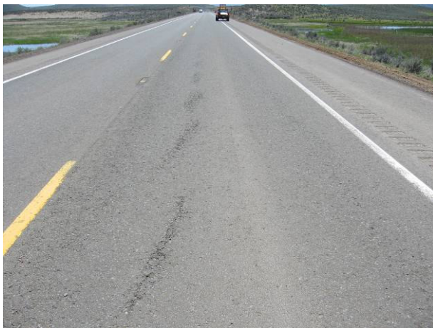
Poor quality construction - segregation
