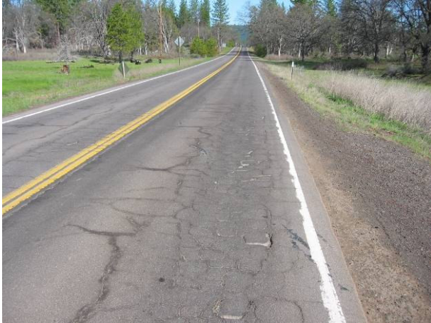
Consistent cracking on selected section
