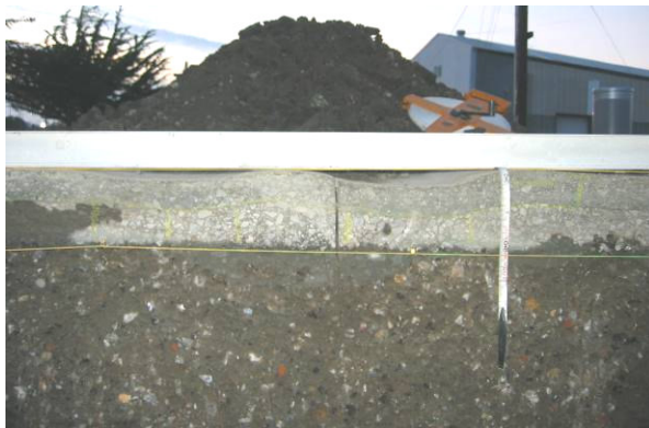
Note rutting in underlying AC layer.
