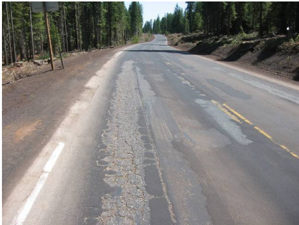
Inconsistent rutting and cracking
