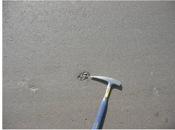
Poor quality construction - contamination
