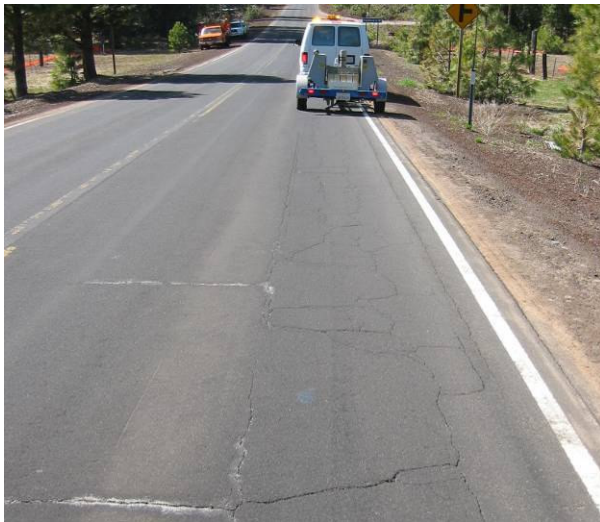
Structural assessment. Note salt in cracks.
