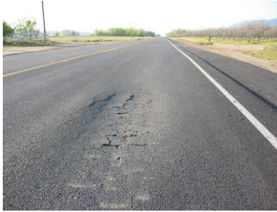
Surface distress in new overlay
