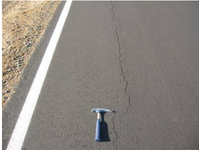
Longitudinal crack in new overlay
