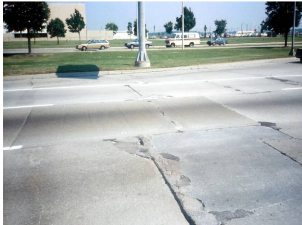
Inconsistent spalling, cracking, and faulting
