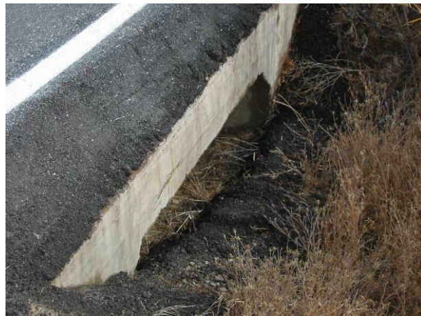
Poor quality construction - drainage impairment
