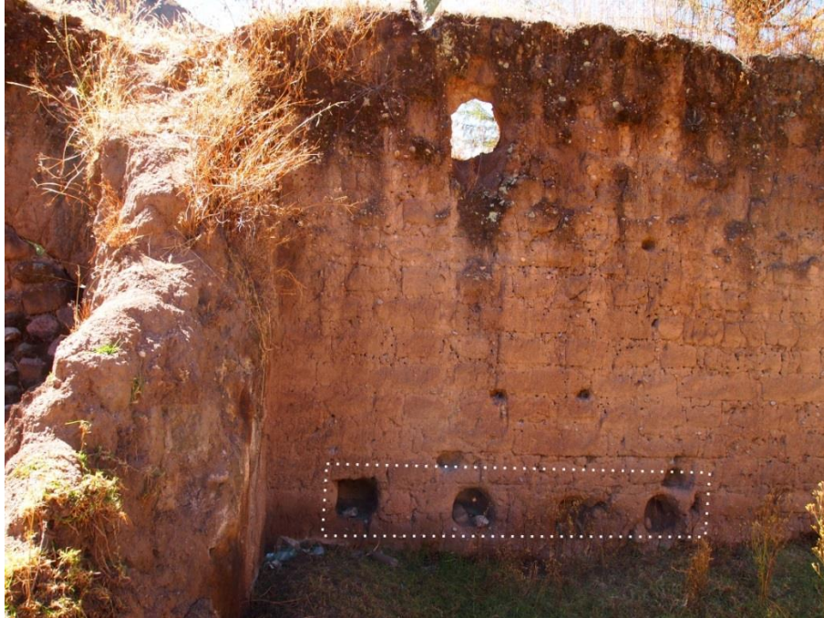
Figure 11.20: Holes for large beams that would have been part of a covering for the depression at the northern side of the room.
