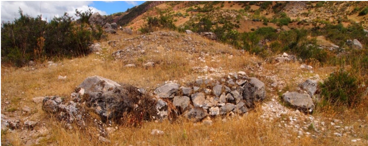
Figure 5.12: Example of a retaining wall, approximately 70cm in height with artificial fill behind it.
