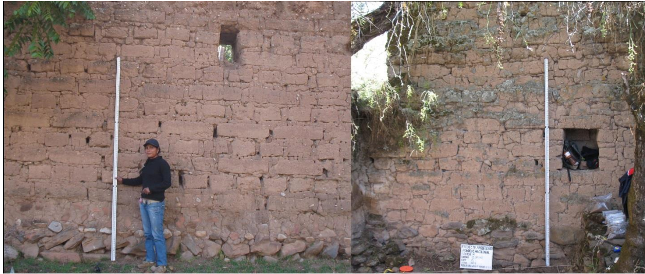
Figure 11.30: Comparison of obraje wall construction (left) with PC15 domestic wall construction (right).
