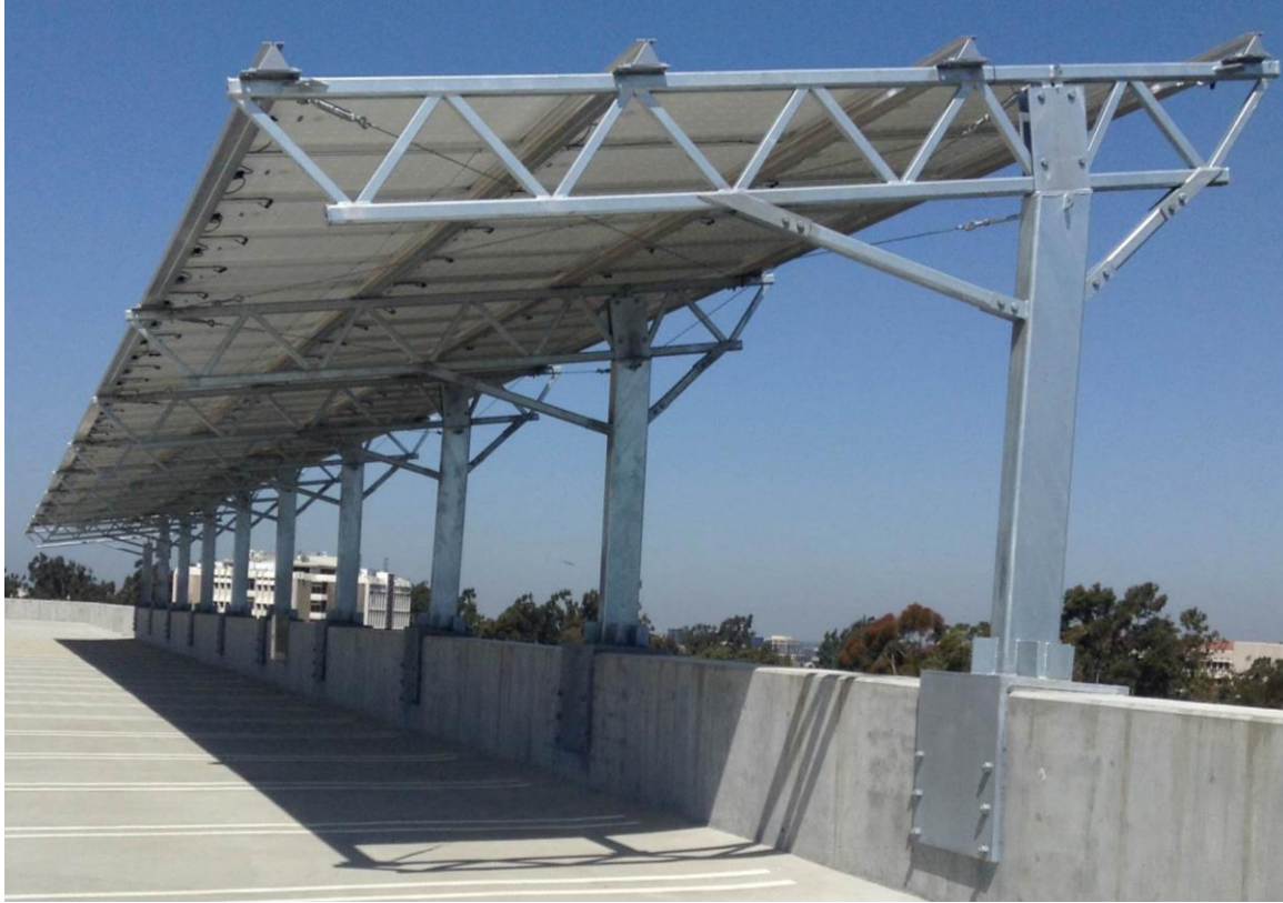
Figure 6: Rooftop solar PV for car shade project (Reyes 2014)
