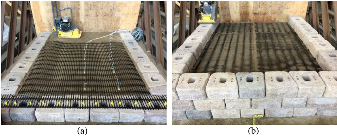
Figure 6.27 Construction of GRS bridge abutment: (a) longitudinal reinforcement layer; (b) transverse reinforcement layer.
